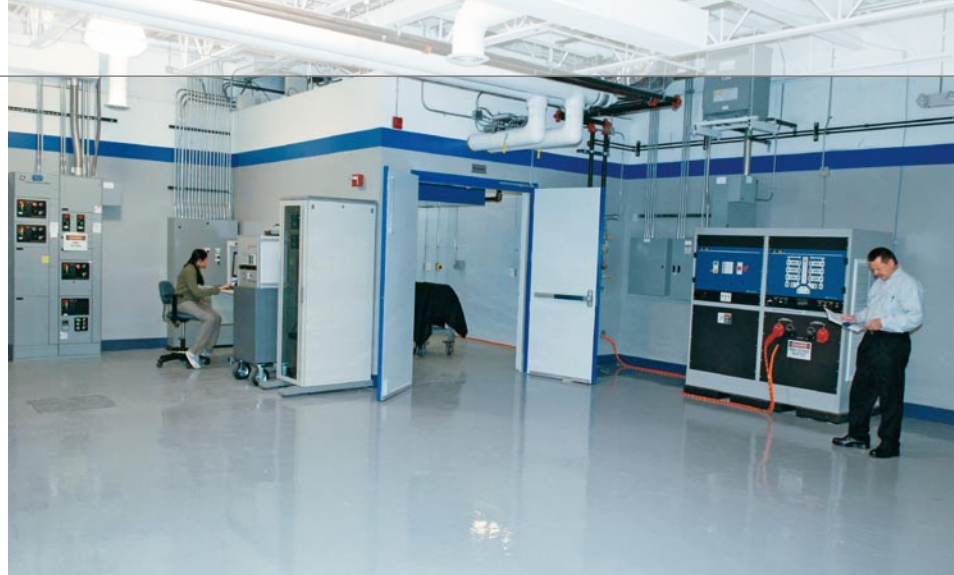
The test chambers are equipped with robust safety and filtration systems – ideal for working with cells and packs using unvalidated support systems.
